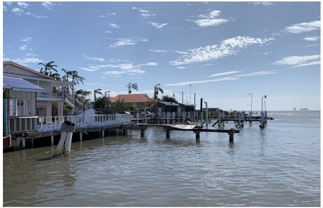
Damaged deck of that old pier
