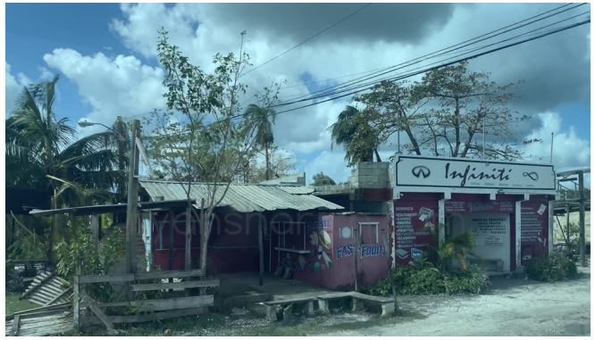
You would see a damaged and abandoned buildings or houses every so often.
