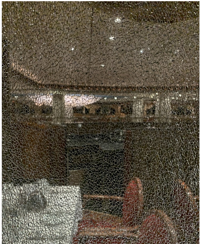
Shattered glass pane next to the restaurant.
